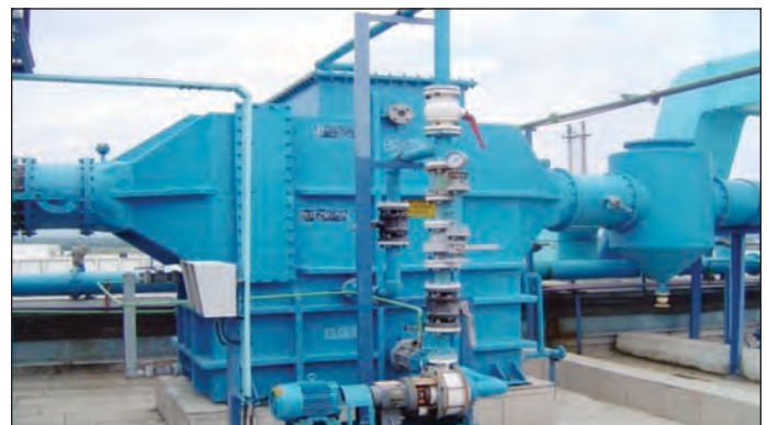
Horizontal scrubbing system.
