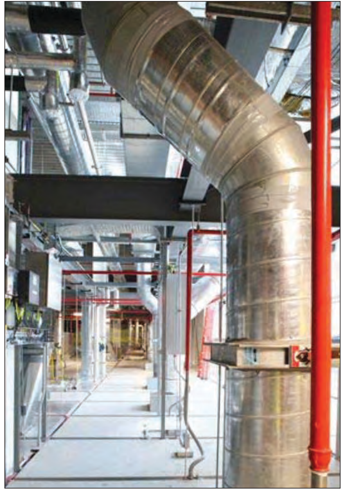
Walkable ceilings minimize traffic in cleanrooms.
