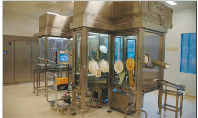
Filling line in the filling room.
