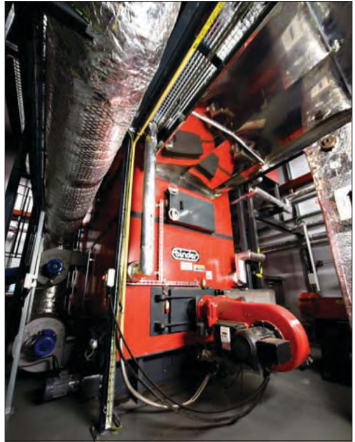
Biomass boiler fueled woodchip from sustainable forests.
