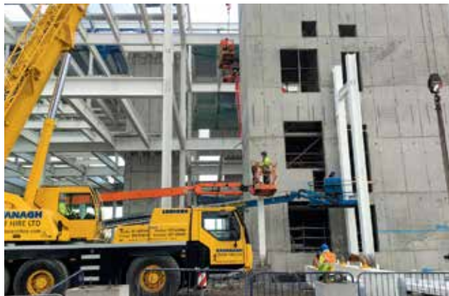
The company is constructing a new state-of-the-art, large-scale biologics manufacturing facility in Cruiserath, County Dublin, Ireland, that will produce multiple therapies for the company's growing biologics portfolio.
