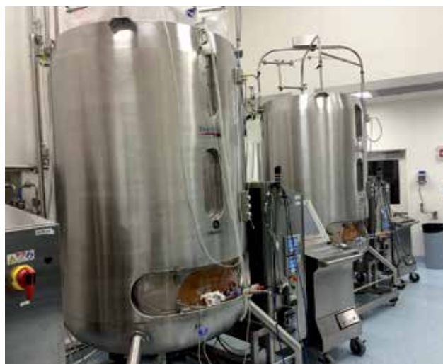
The company's new multi-host, multi-product, small-scale single-use biologics facility in Bothell, Washington
