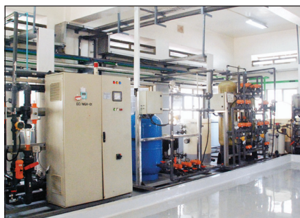
Eisai Pharmatechnology & Manufacturing Pvt. Ltd.: water pretreatment.
