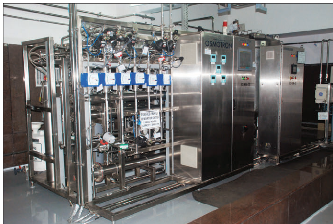
Purified water system.
