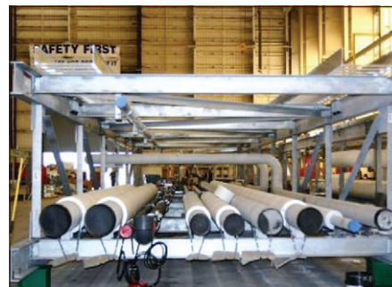
Merck & Co., Inc.: interior pipe rack module.
